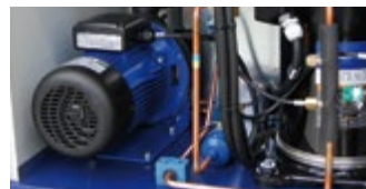
Pump P3 (3 barg) / P5 pump (5 barg, optional).
